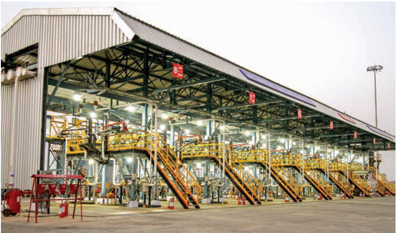
Flame proof LED lighting at tank truck loading gantry at one of our POL locations
